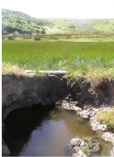
P-070: Headcut up spillway into exterior dam face.
