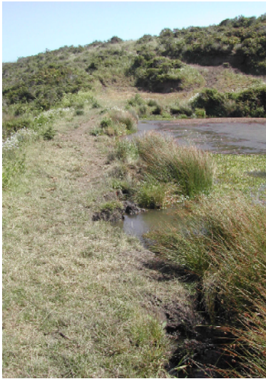
P-071: Wave erosion along interior dam face.
