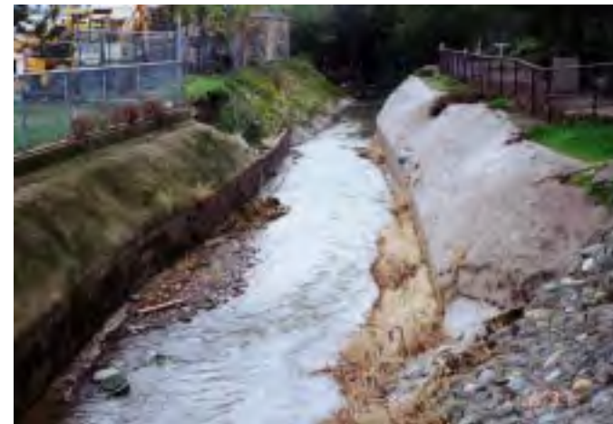
(Photo 31) Looking downstream at revetted channel at Davis Park, which floods with flows that have a recurrence interval of less than 10 yrs. This area is represented by cross section "K" in Figure 49 (see facing page).
