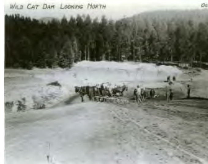
(Photo 19) Construction underway at Wildcat Reservoir (Jewel Lake) 1919. Consider the amount of sediment production and downstream impacts from these disturbed soils. Channel incision downstream of the dam and subsequent sediment production has been ongoing. Source: East Bay Regional Park District.
