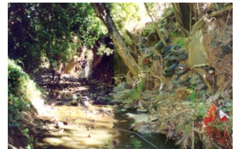
(Photo 40) Non-engineered revetment is failing into Wildcat Creek.
