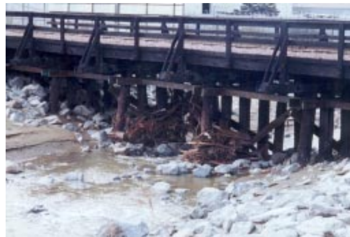
(Photo 55) Floating woody debris collects on the railroad trestle piers. The beams and the trestle impede the passage of flood flows and contribute to the formation of backwater floods. Flows have exceeded the top of the tracks.
