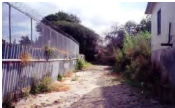
(Photo 30) Looking upstream from the Rumrill box culvert at the plain bed of the creek that lacks topography. This reach is represented in cross section "I" (which is drawn looking downstream) in Figure 49.
