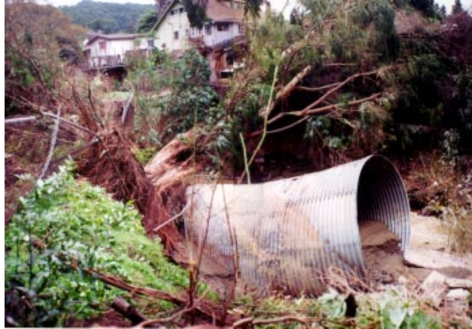
(Photo 3) A deteriorated 15 ft diameter culvert fails along with its overlying fill in the Upper Alluvial Plain Segment, January 1997.
