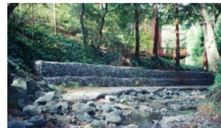
(Photo 41) A new wire basket gabion and apron revetment in McBryde Reach, January 1998.
