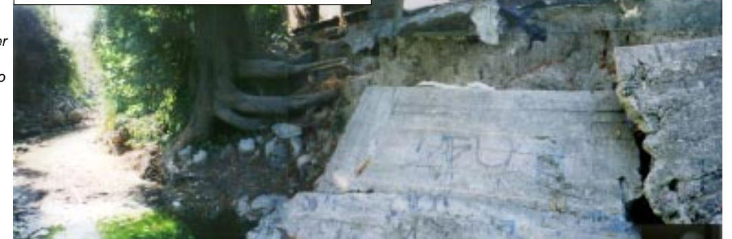
(Photo 44) August 1998, a concrete revetment collapses along the Upper Alluvial Plain.
