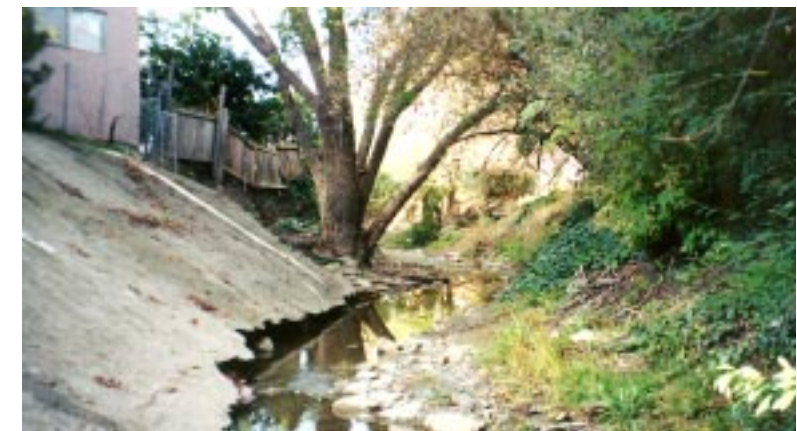
(Photo 38) A revetted bank and a natural bank oppose each other along the Alluvial Plain. Bed incision within the last 50 years is apparent along the base of the concrete and at the exposed roots on the right bank.
