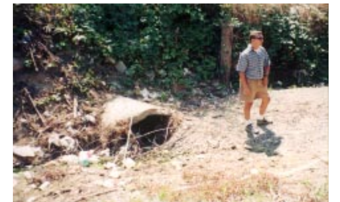
(Photo 56) A buried reinforced concrete pipe gives evidence of an aggraded bed. It is located near station 6200 on Figure A above.
